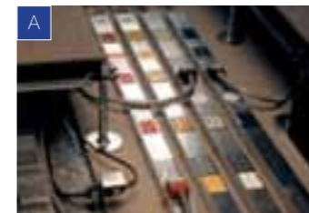
CMS: Cable Management System
